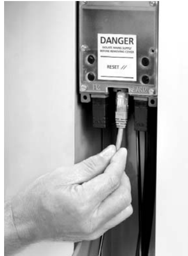
Connecting the PC to the controller
